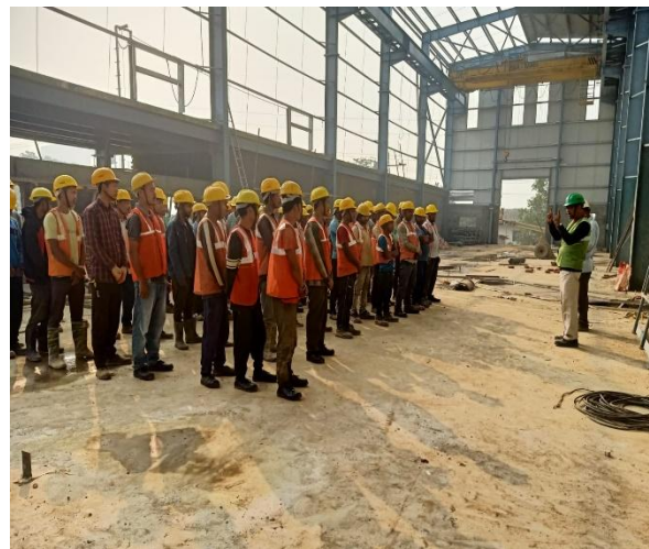
Photo Plate 10: GBV and SH at Sonapur S/S (Pkg-H).
