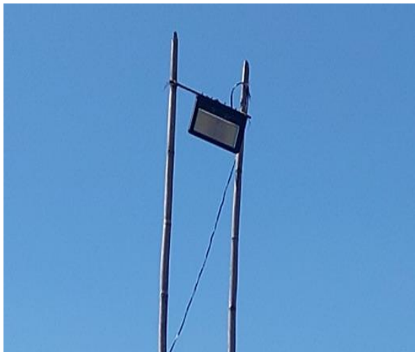
Photo Plate 19 – Adequate lighting facility provided at Chhaygao T/L
