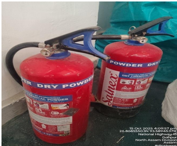
Photo Plate 25 - Fire extinguisher available at Gohpur substation.
