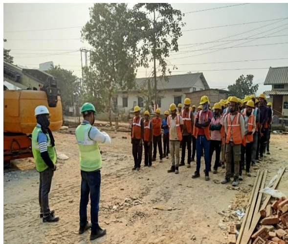
Photo Plate 9: GBV and SH at Sonapur S/S (Pkg-H).
