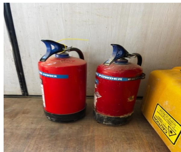
Photo Plate 20 – Adequate fire extinguishers have been installed at Khumtai substation.
