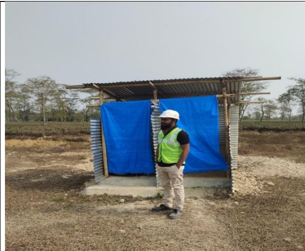
Photo Plate 8 – Toilet facilities for workers provided at Khumtai S/S
