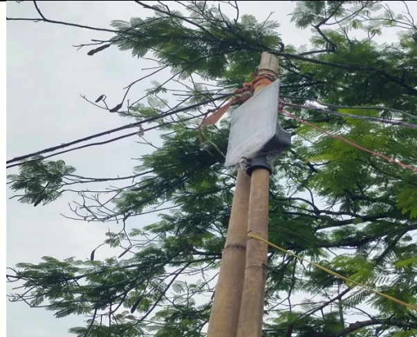
Photo plate 51 – Lighting facility provided at Gohpur S/S
