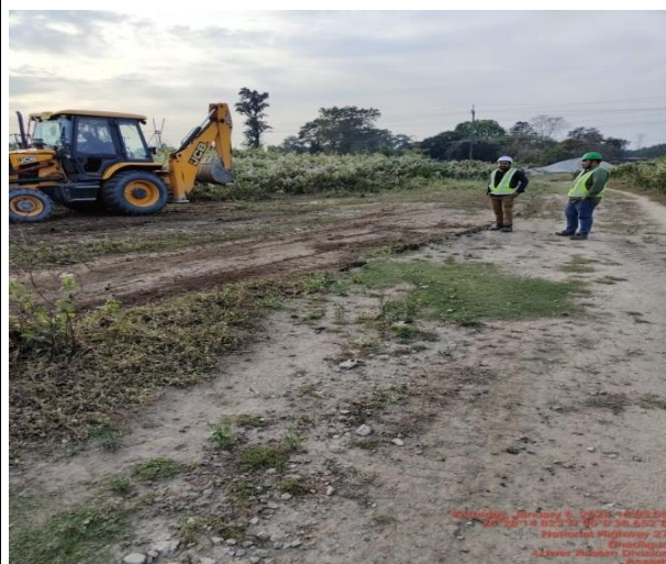
Photo Plate 9 – Unwanted bushes are trim down around the Agomoni substation area.
