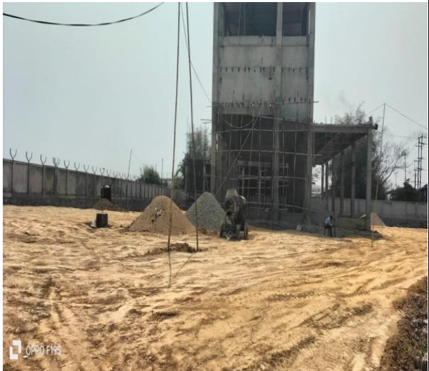
Photo Plate 22 – Work stopped due to non availability of manpower at Chhaygaon S/S
